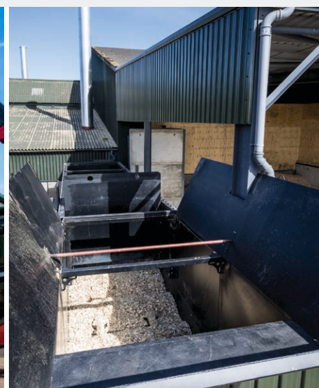
Dryer moving floor
