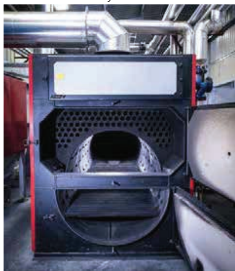
SASP System 1 MW
