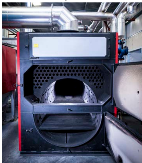
SASP System 1 MW
